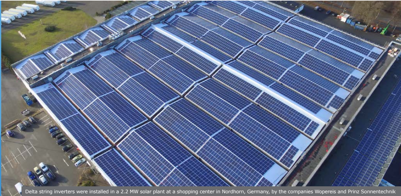
Delta string inverters were installed in a 2.2 MW solar plant at a shopping center in Nordhorn, Germany, by the companies Wopereis and Prinz Sonnentechnik
