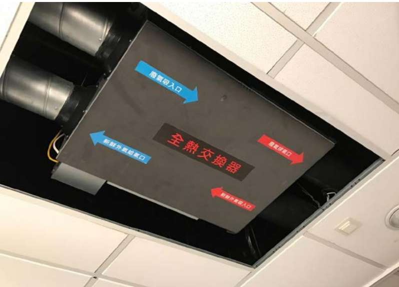
Besides helping energy conservation and carbon reduction, green buildings also make use of the heat exchange system to maintain indoor air quality (Image provided by: Evan Kao)
