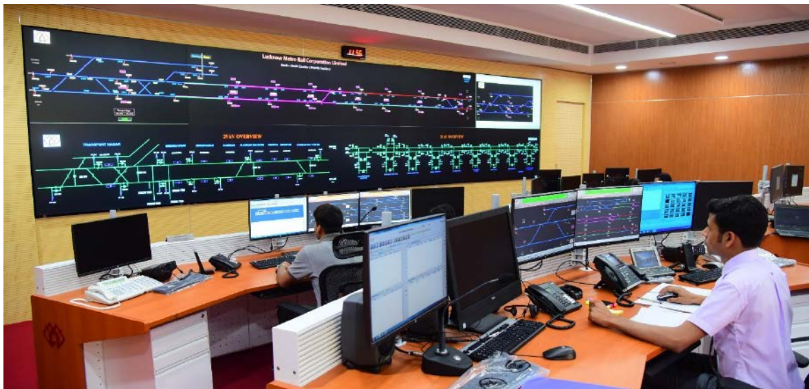
Delta's brightest video walls at Lucknow Metro MRTS
