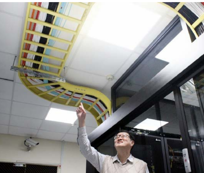
The cables of the data center are colored on purpose
