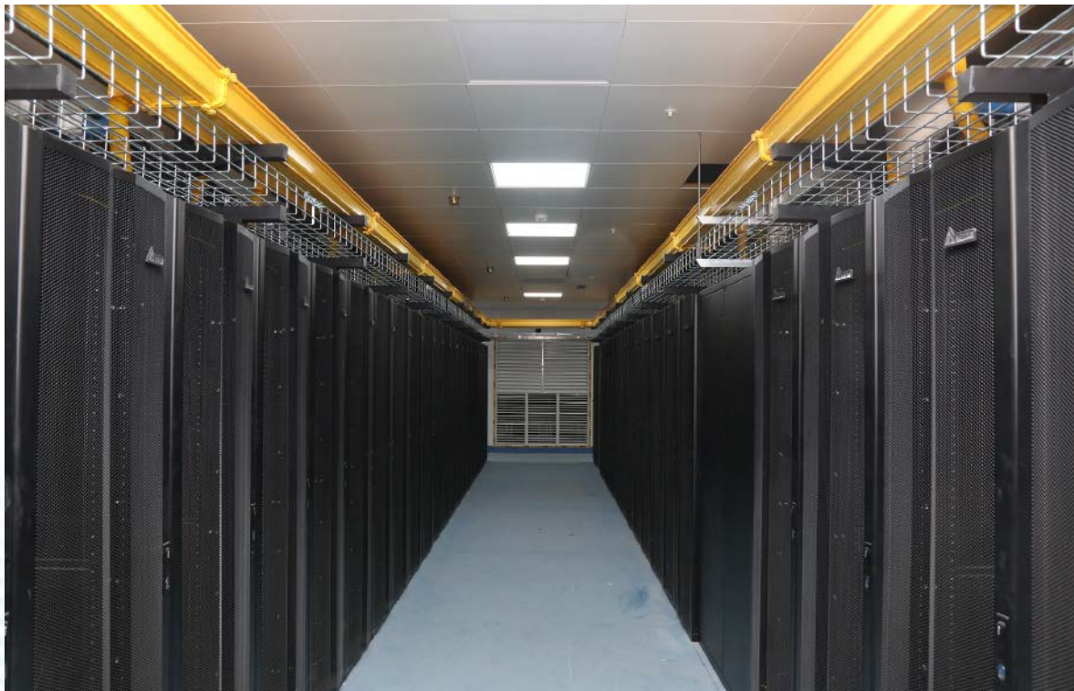
Delta has deployed 10 micro-module rooms for its premade micro-module data center solution in the first phase of the project
