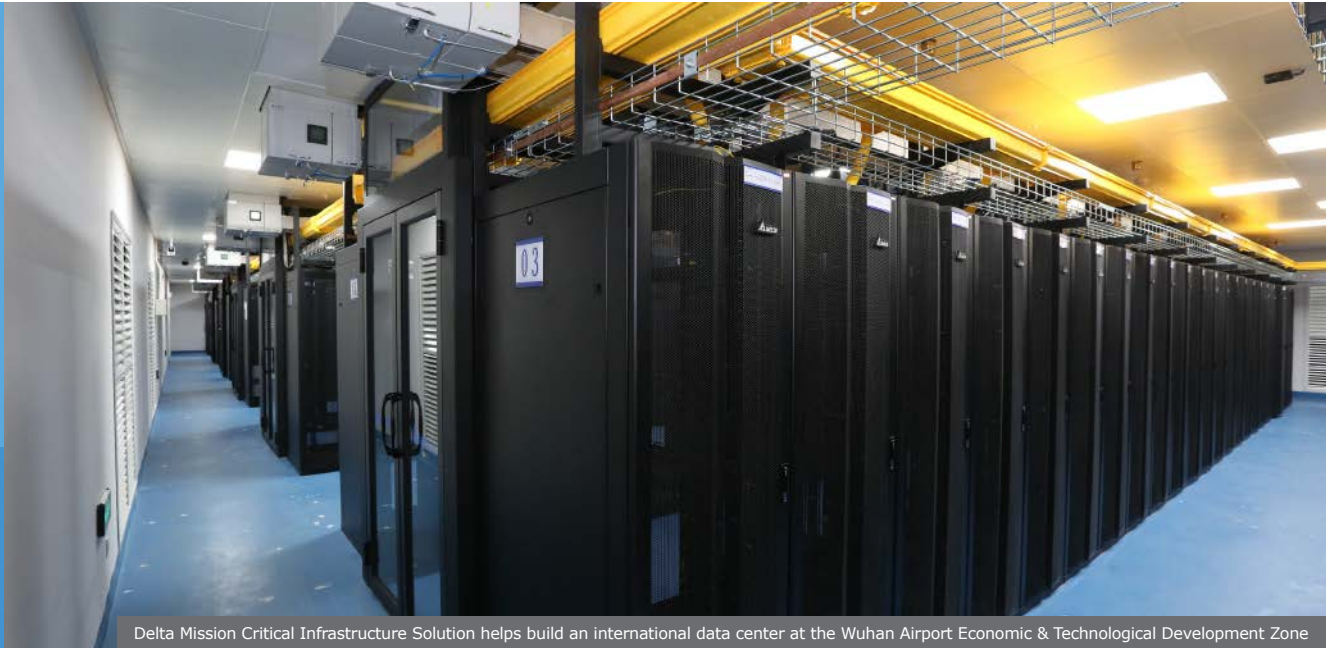
Delta Mission Critical Infrastructure Solution helps build an international data center at the Wuhan Airport Economic & Technological Development Zone
