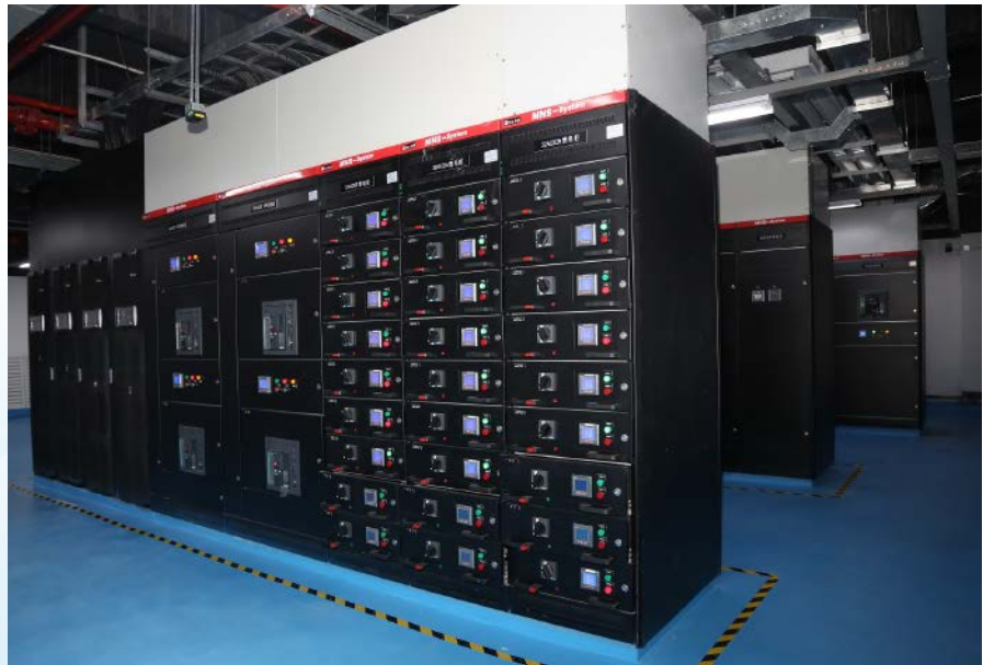
In response to the 5A challenge, Delta utilizes its DPH 500kVA Series UPS, which is designed for ultra-large-scale IDCs, employs the latest technologies, and has the highest power density in the industry
