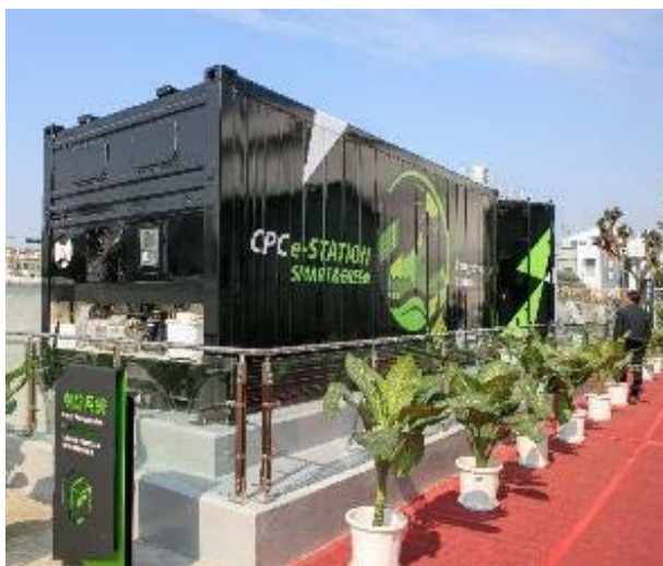
The Delta ESS installed at the CPC Smart Green Energy Station demonstration site seen at the opening of the station
