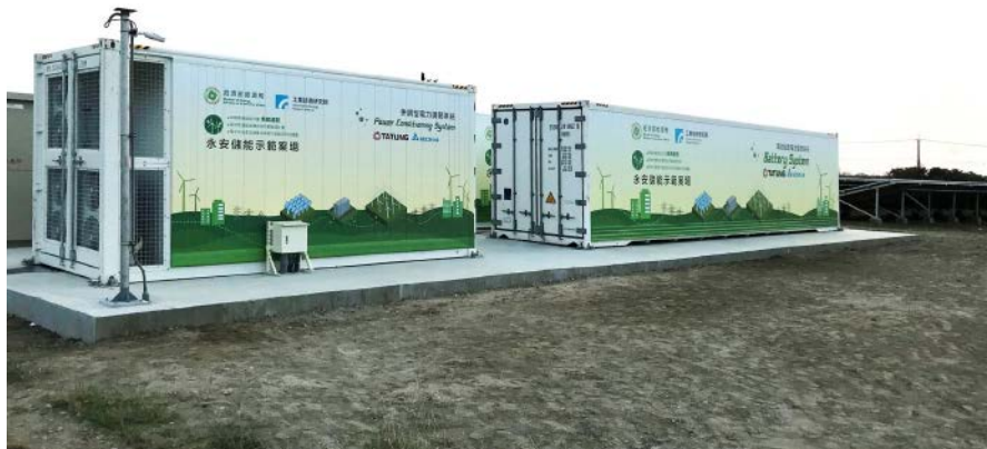
ESS installed at the Kaohsiung Yongan PV plant
