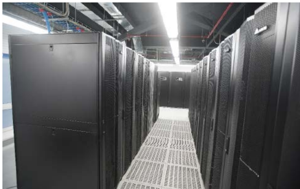
Delta offers integrated data center solutions to a leading mining company's four data center sites with a total of 365kW power capacity
