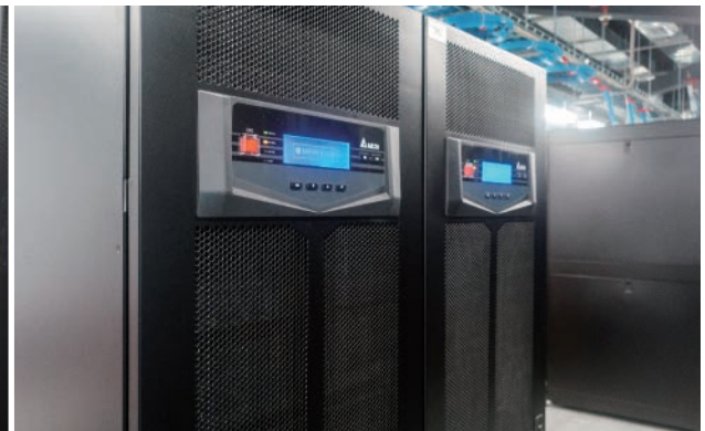
Delta's Ultron HPH series online UPS are installed to protect IT equipment and precision cooling systems in the data centers
